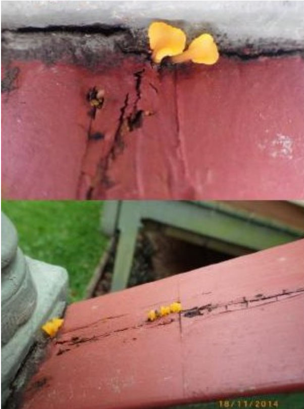
Figure 1. Wooden stair handrail with decay and fruiting bodies.
